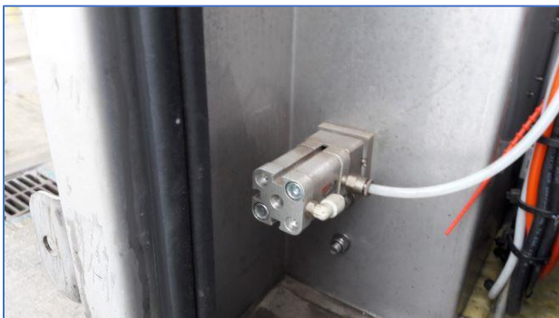
Pneumatic valve to operate airlock
